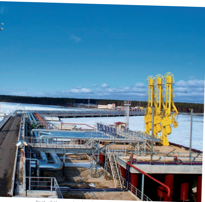
Part of the marine loading station at Primorsk Commercial Sea Port
