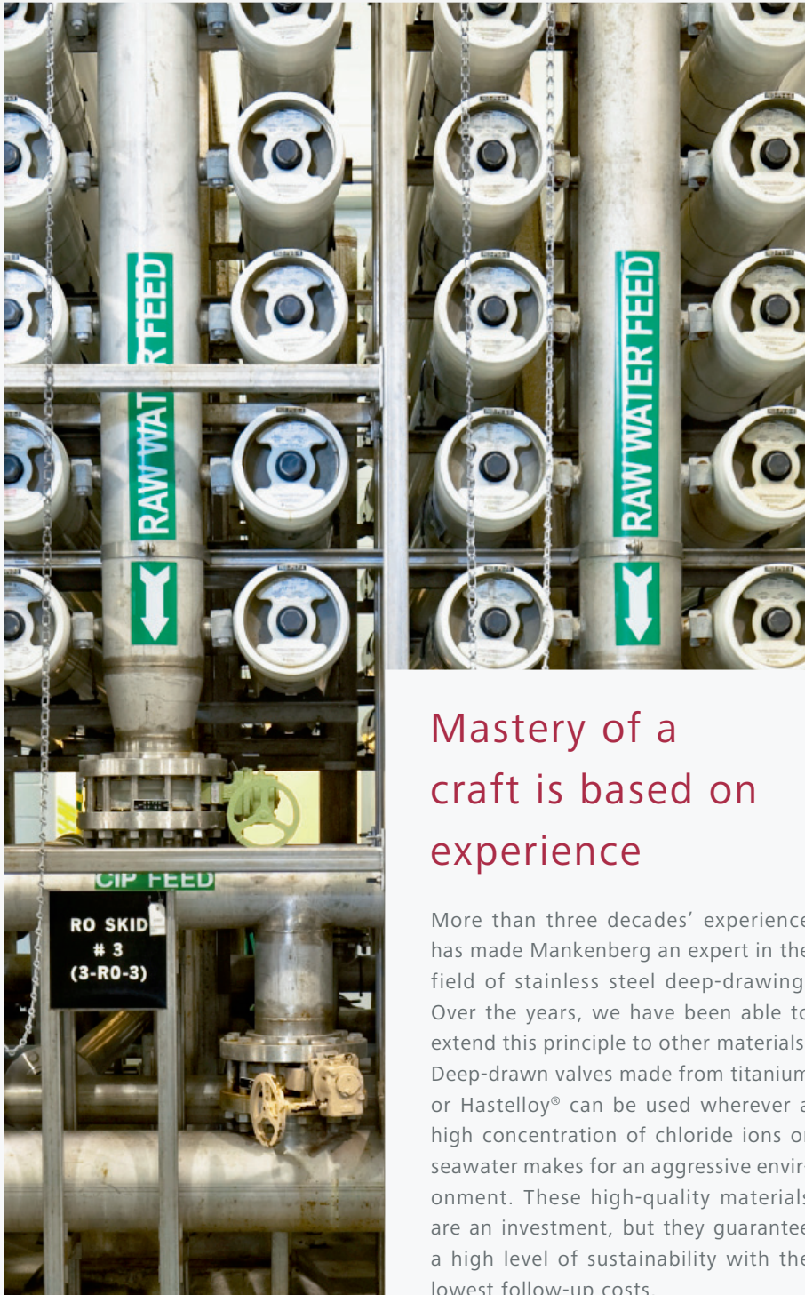
Detailed view of a seawater desalination plant
